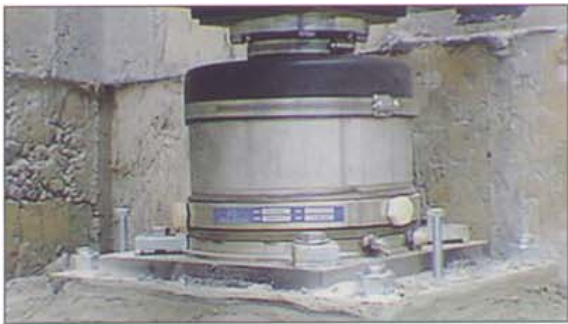
The close-up view of one of the Emery Winslow Model 136, 75,000-pound hydrostatic load cells used in the Bocker Grain installation. (Photo courtesy of Midwest Scale Company, Rockford, Ill.)
