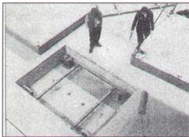
Installing one of the nine Emery Winslow weigh platforms in Boeing's painting facility hanger.
